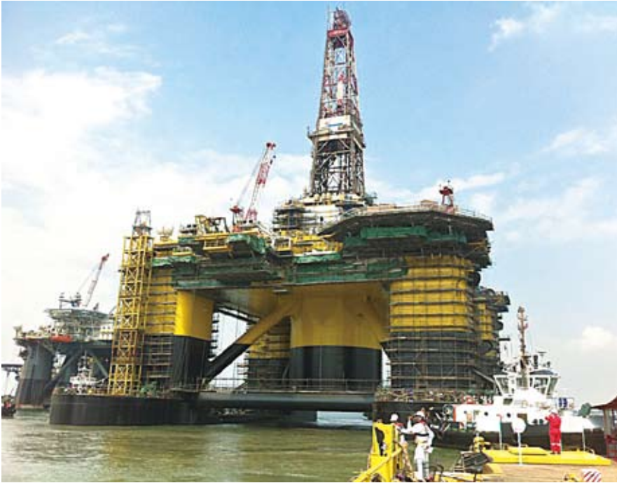
Repair on the semi Jack Bates was completed safely and on time
