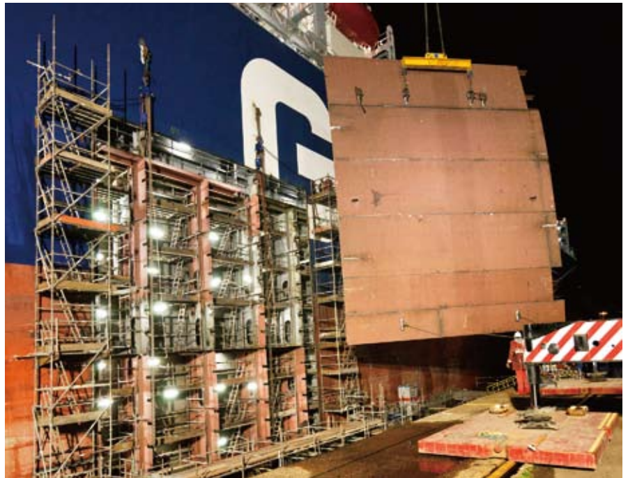
Keppel Verolme renewed 44 tonnes of steel and applied a complete paint job, all within 16 days, on container vessel CMA CGM Alaska
